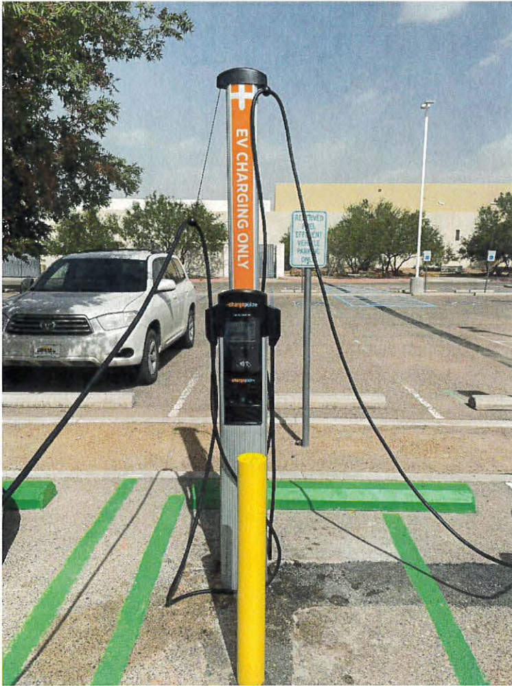
Las Cruces Conventional Center 2 chargers installed
